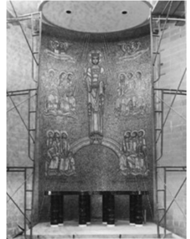
The mosaic and altar under construction in Immaculata Chapel in Heiss Hall titled "Christ King."
