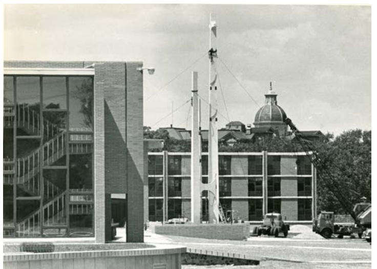
The seminary under construction, with the dome of Henni Hall in the distance.
